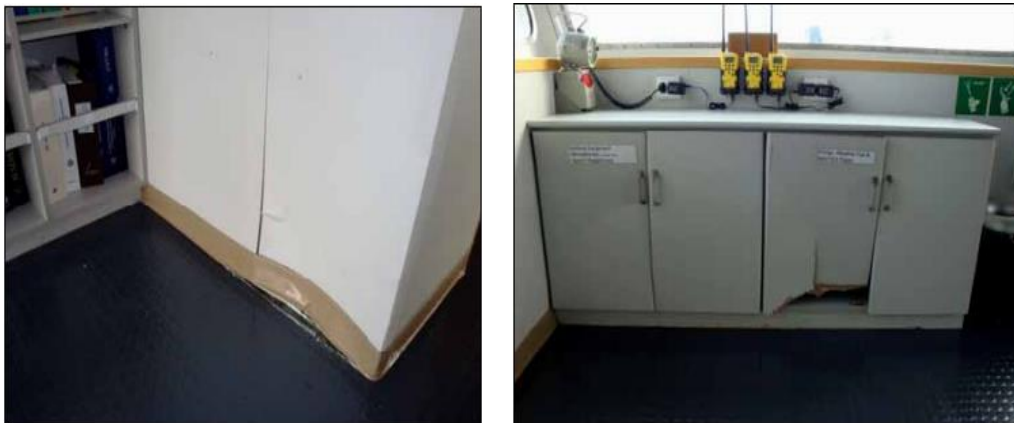
Figure 3.11: Impact damage and deformation of interior[13]
