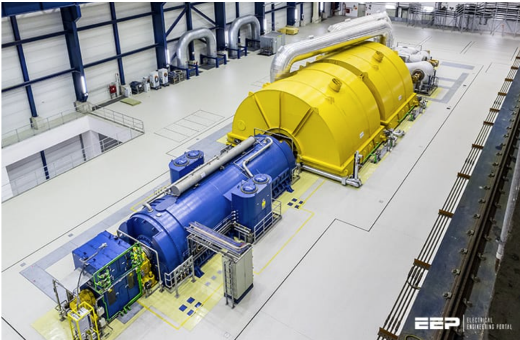
FIGURE 1.1: Alstom's "ultra-super-critical" steam turbine at the Boxberg power plant in Germany can produce 600MW (credit:GE).
