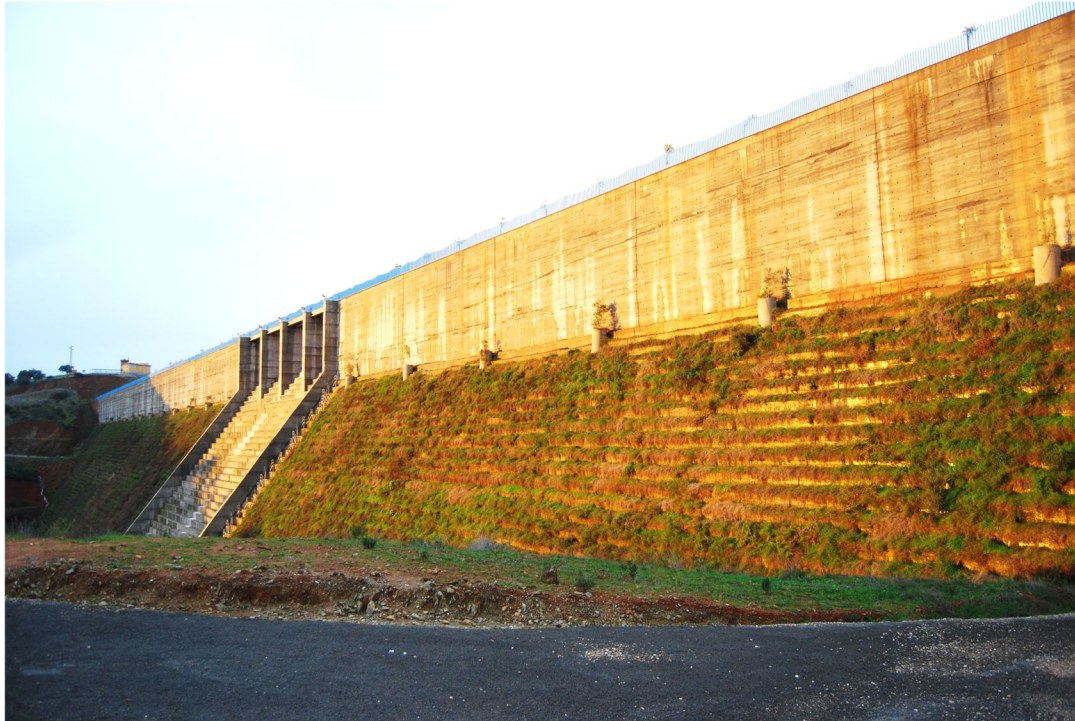
Figure 18. Example of dam with planted downstream face - La Breña II (Spain). Image source: https://lh5.googleusercontent.com/p/AF1QipMy-5InliGbt4FyZqMJG1GdY73tAet1oodIPGB=h1440
