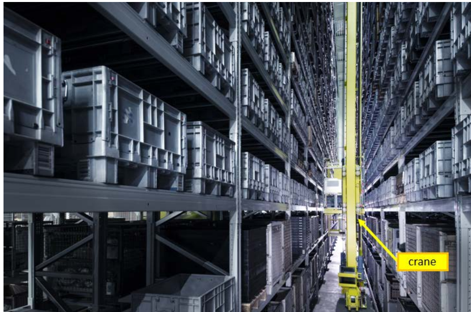
Figure 2.7: Example of a mini-load automated racking system (photo courtesy of Nedcon B.V.).
