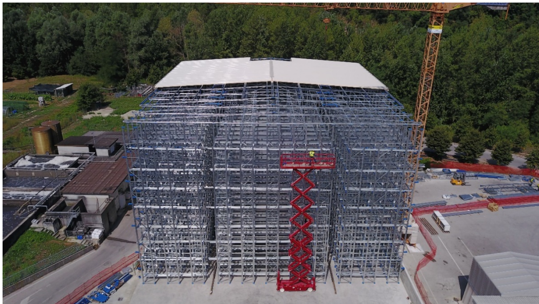
Figure 2.6: Example of a multi-depth ARSW in the construction stage (photo courtesy of SACMA S.p.a.).
