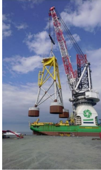
Figure 2-23 Suction bucket jacket being picked up by heavy lift jack-up vessel ( www.maritimejournal.com )
