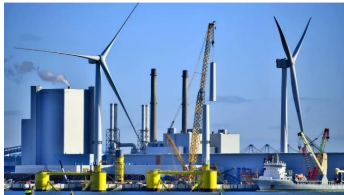
Figure 2-43 Wind turbines being mounted on semi-submersible foundations for Kincardine Offshore Wind Farm ( www.principlepower.com )
