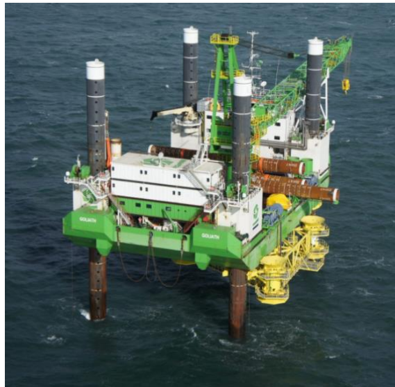
Figure 2-28 Pre-piling template for the Borkum West II Offshore Wind Farm tripods (twd.nl)
