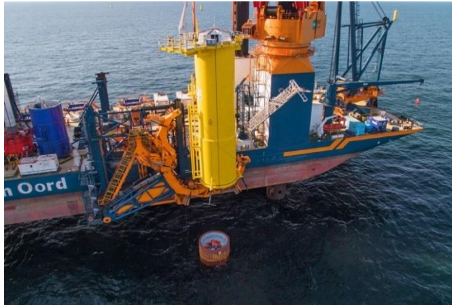
Figure 2-10 Transition piece being lowered into position at the Gemini Offshore Wind Farm ( www.gemini.com )
