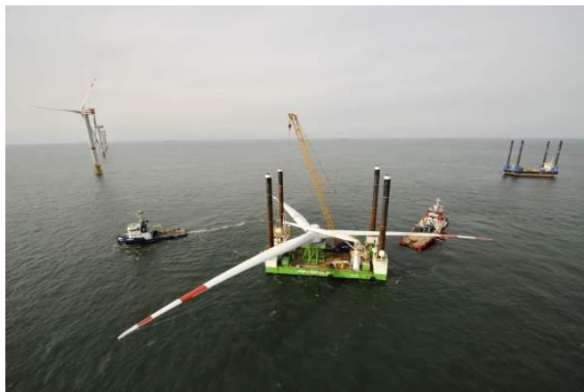
Figure 2-12 Pre-assembly of nacelle and blades for the Thornton Bank Offshore Wind Farm ( www.repower.com )
