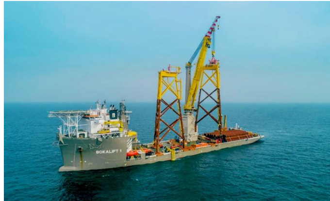
Figure 2-17 Jackets being installed on piles for the East Anglia One Offshore Wind Farm ( www.heavyliftnews.com )
