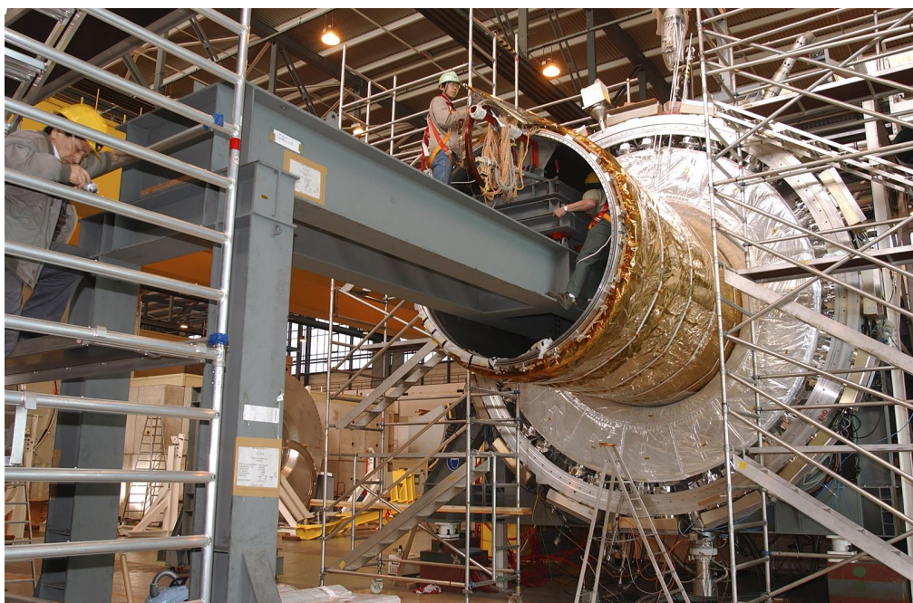
Figure 2.3: ATLAS Central Solenoid magnet during installation.
