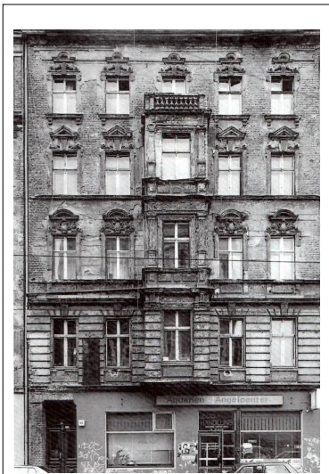
Picture 3.15: The house on number 46 before the repairs
