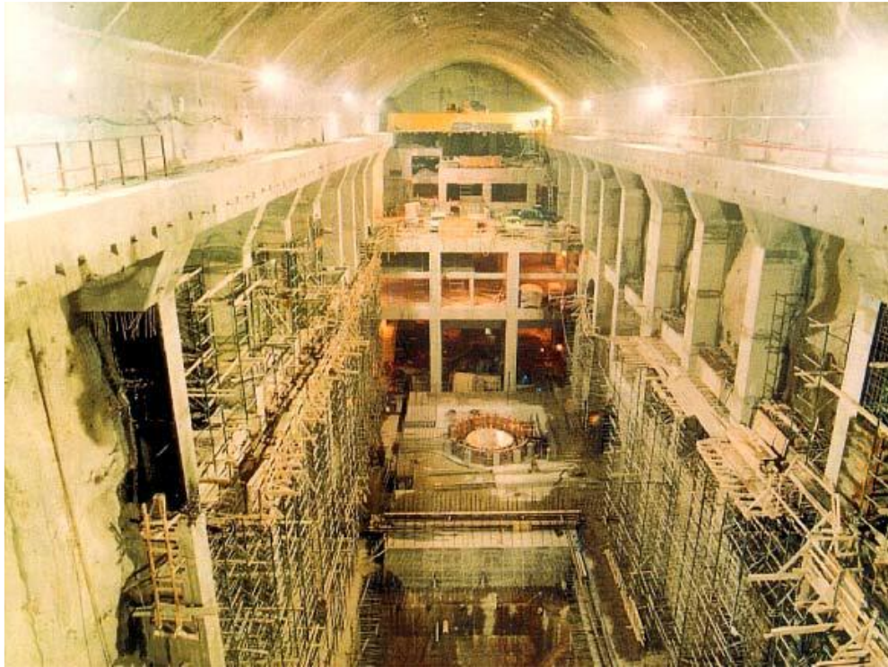
Figure 5 The Underground Cavern of the Hydroelectric Power Plant in Thisavros, Greece (Source: Kaliampakos, 2009).
