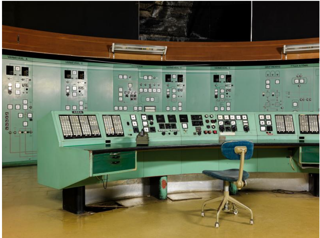
Figure 23 The control room in Agesta (Source: https://history.vattenfall.com/stories/agesta-power-plant ).
