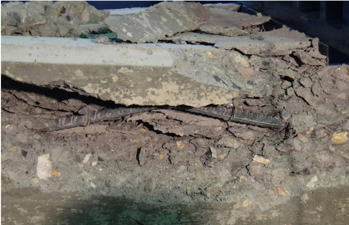
Fig. 5.40- S5- Buckling of longitudinal rebar at the end of the test (fig. 5.42 and 5.43, points D and D')
