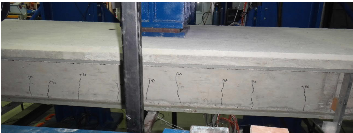
Fig. 5.166- S10- Cracks at deflection of 25 mm (fig. 5.172 and 5.173, points B and B')
