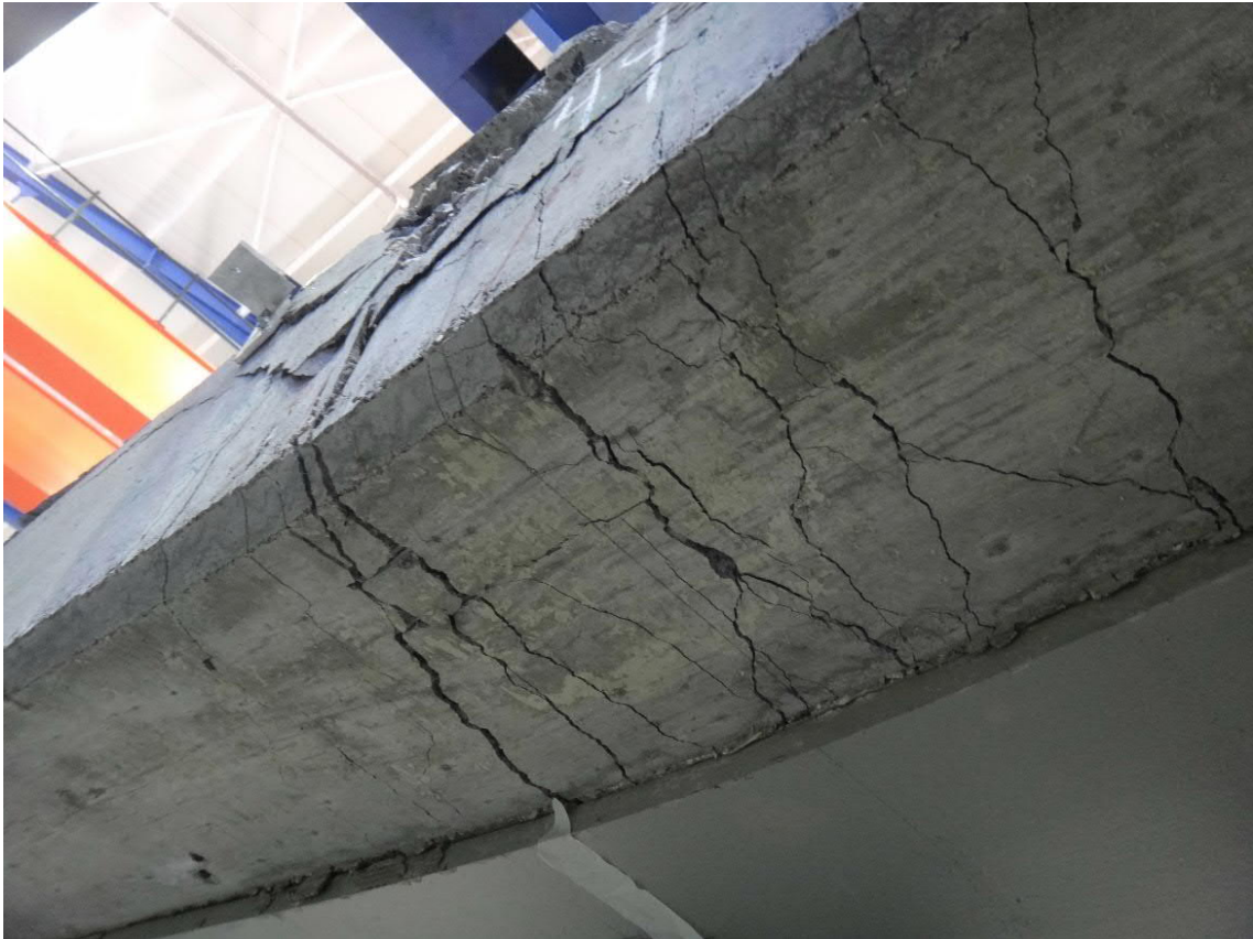
Fig. 5.100- S6a- Cracking of the specimens bottom and sides at the end of the test (fig. 5.104 and 5.105, points D and D')
