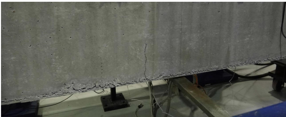
Fig. 5.64- S11- Hair-line cracks at deflection of 18 mm (fig. 5.71 and 5.72, points A and A')
