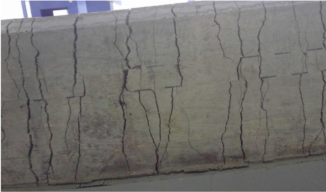
Fig. 5.142- S8- Bottom of concrete plate at the end of the test (fig. 5.144 and 5.145, points G and G')
