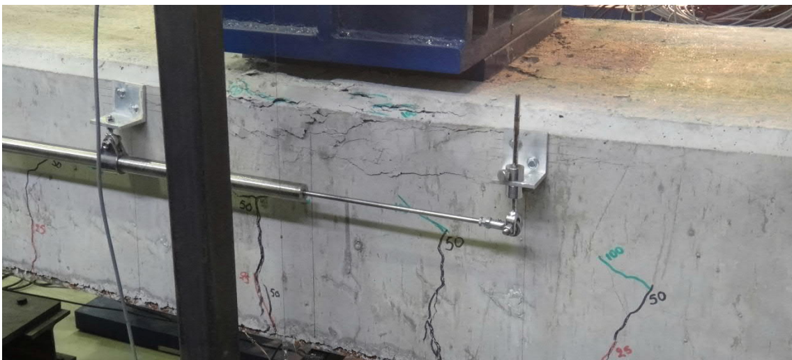
Fig. 5.39- S5- Compressive cracks at deflection of 105 mm (fig. 5.42 and 5.43, points C and C')
