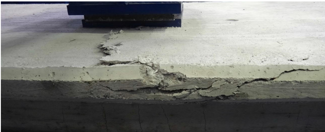
Fig. 5.168- S10- Cracks at the top of the concrete (fig. 5.172 and 5.173, points D and D')
