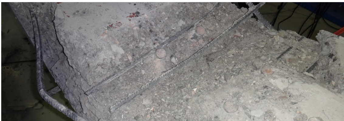
Fig. 5.4- S2- The beam top mid span at the end of the test (fig. 5.6 and 5.7, points D and D')
