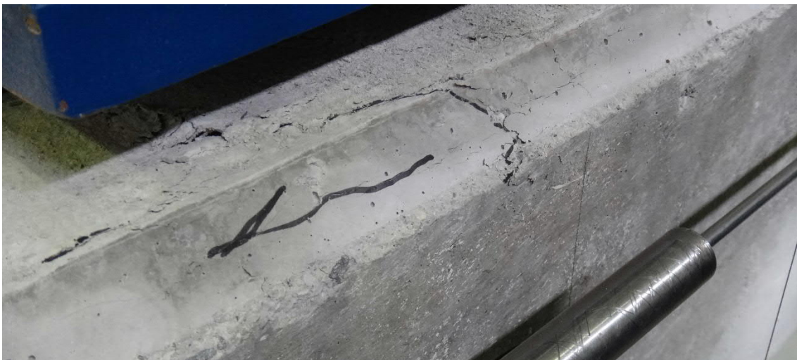
Fig. 5.15- S3- Compressive cracks at deflection of 105 mm (fig. 5.18 and 5.19, points C and C')
