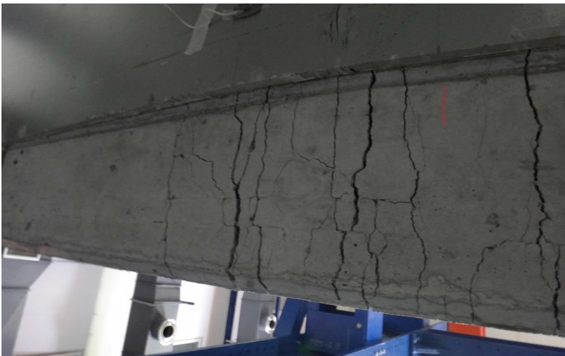
Fig. 5.129- S7- Cracks at the bottom of concrete plate at the end of the test (fig. 5.130, point F)
