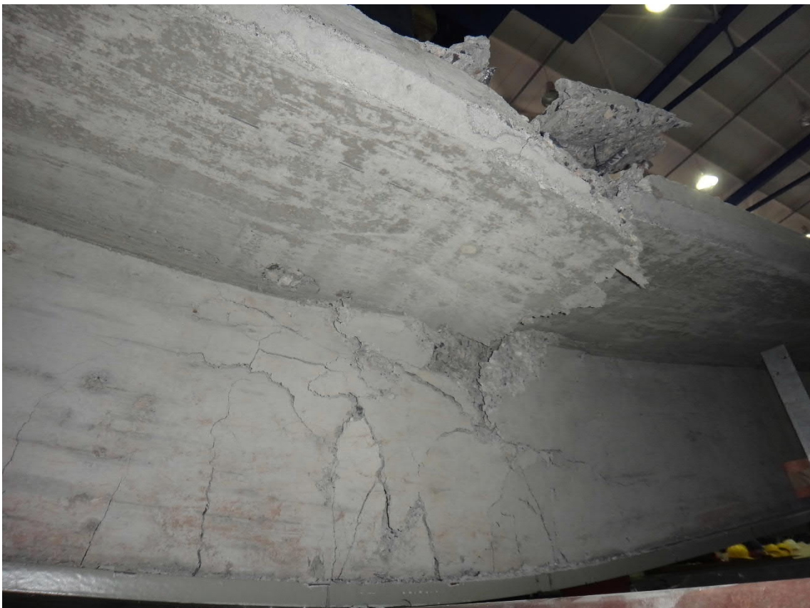
Fig. 5.158- S9- Cracks at the middle of the span at the end of the test (fig. 5.159 and 5.160, points F and F')
