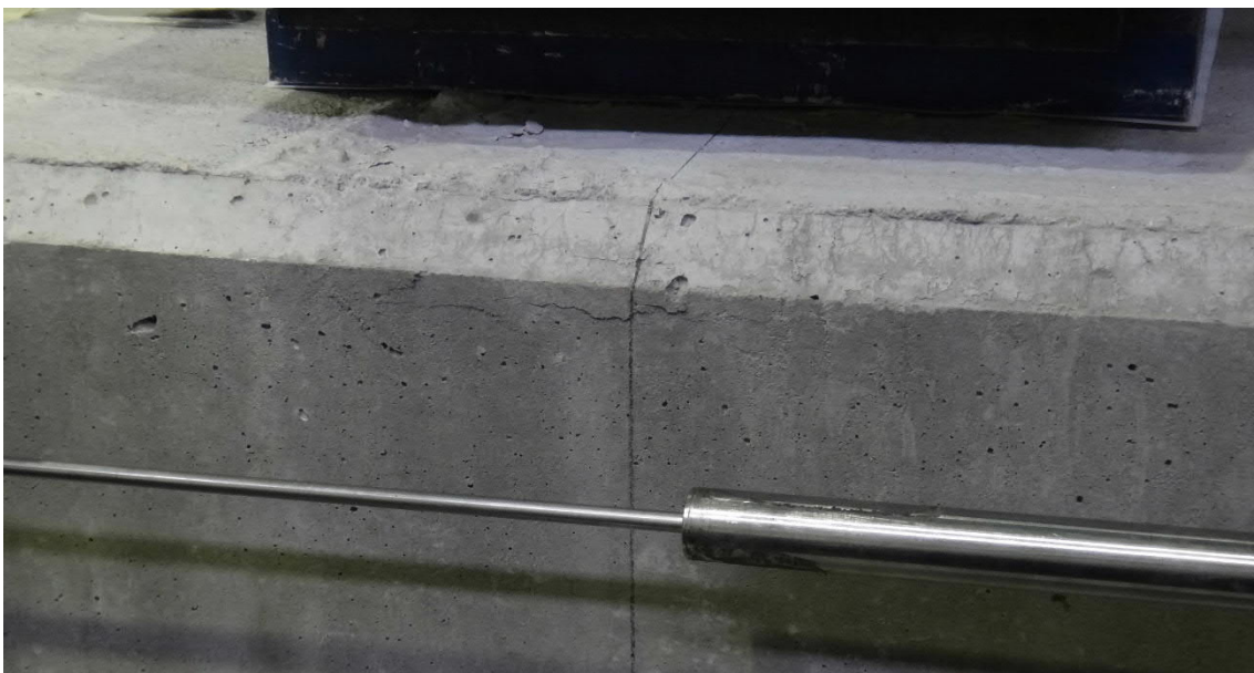
Fig. 5.67- S11- Cracks due to compression at deflection of 65 mm (fig. 5.71 and 5.72, points D and D')
