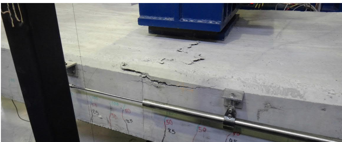
Fig. 5.114- S6b- Cracks at the top face of concrete (fig. 5.117 and 5.118, points D and D')
