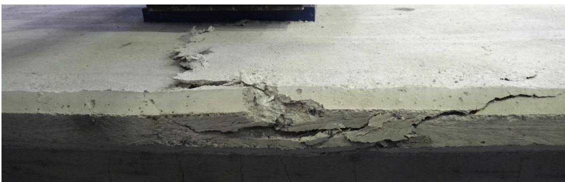
Fig. 5.156- S9- Cracks at the top face of concrete (fig. 5.159 and 5.160, points E and E')
