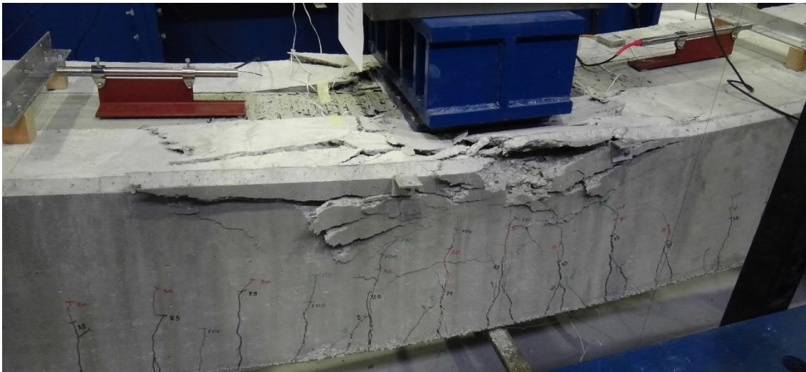
Fig. 5.69- S11- Cracks at deflection of 150 mm (fig. 5.71 and 5.72, points F and F')
