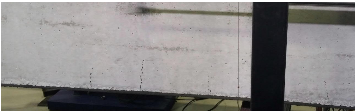
Fig. 5.135- S8- Hair-line cracks at deflection of 19 mm (fig. 5.144 and 5.145, points A and A')
