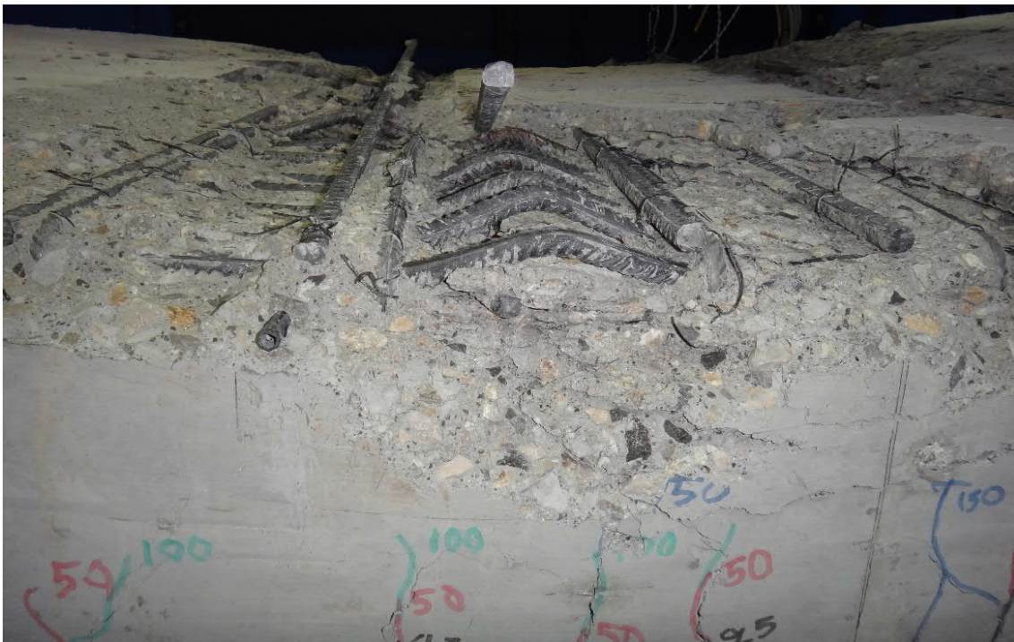
Fig. 5.116- S6b- The beam after the removal of loose concrete (fig. 5.117 and 5.118, points F and F')
