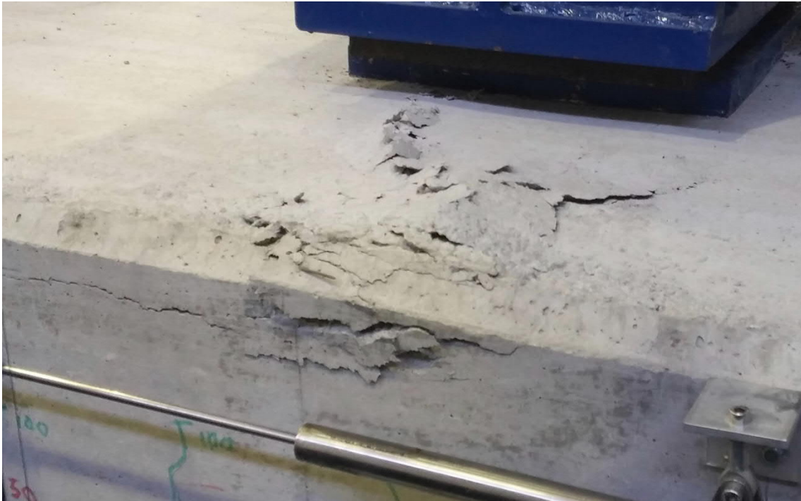
Fig. 5.140- S8- Cracks at the top face of concrete (fig. 5.144 and 5.145, points D and D')
