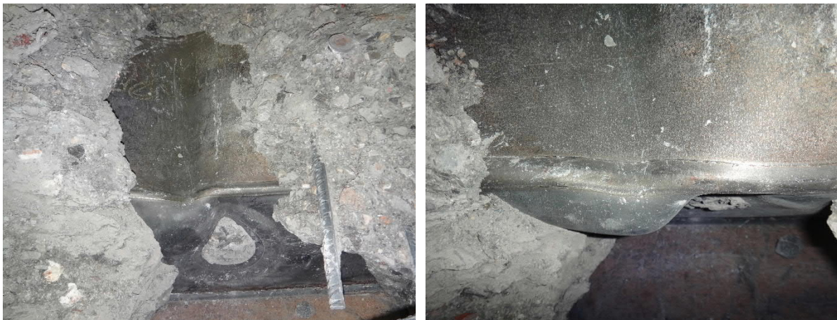
Fig. 5.17- S3- Buckling at the top plate of the steel beam
