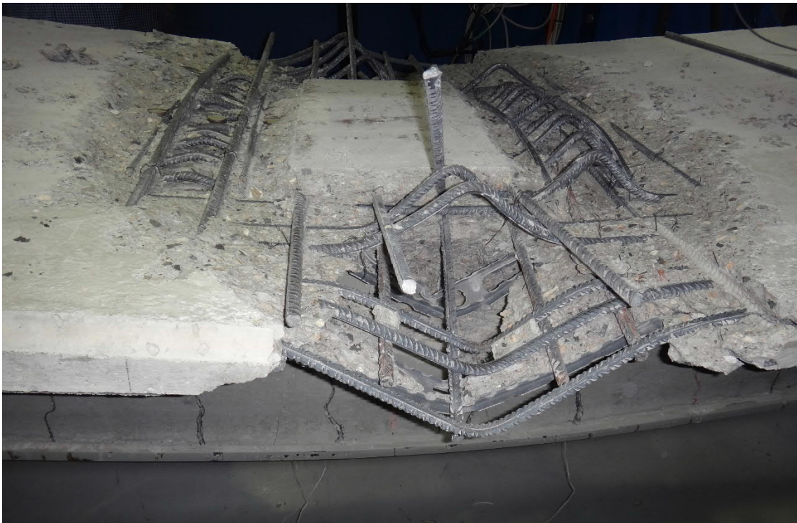
Fig. 5.171- S10- The beam after the removal of loose concrete (fig. 5.172 and 5.173, points E and E')
