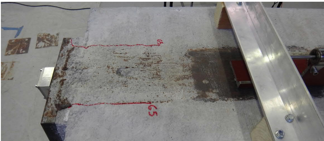
Fig. 5.54- S1- Cracks between concrete and steel at 65 mm deflection (fig. 5.57 and 5.58, points C and C')
