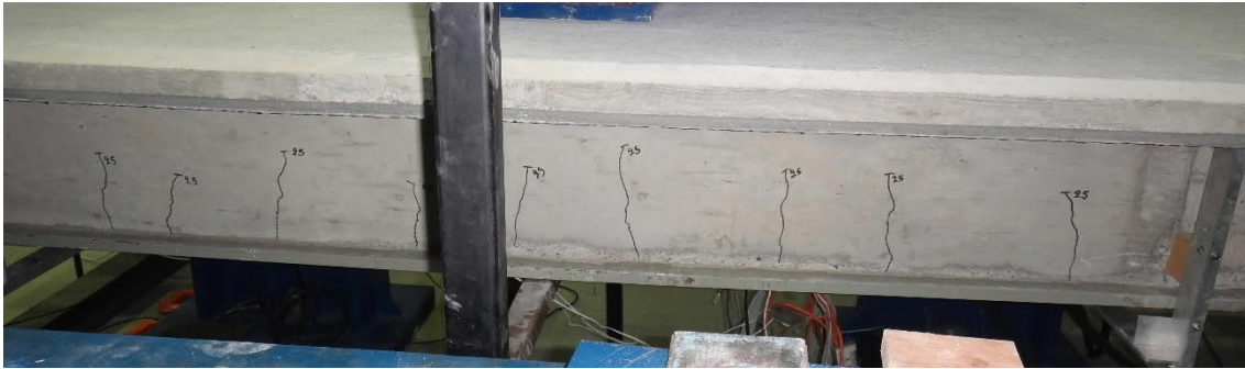
Fig. 5.153- S9- Cracks at deflection of 25 mm (fig. 5.159 and 5.160, points B and B')
