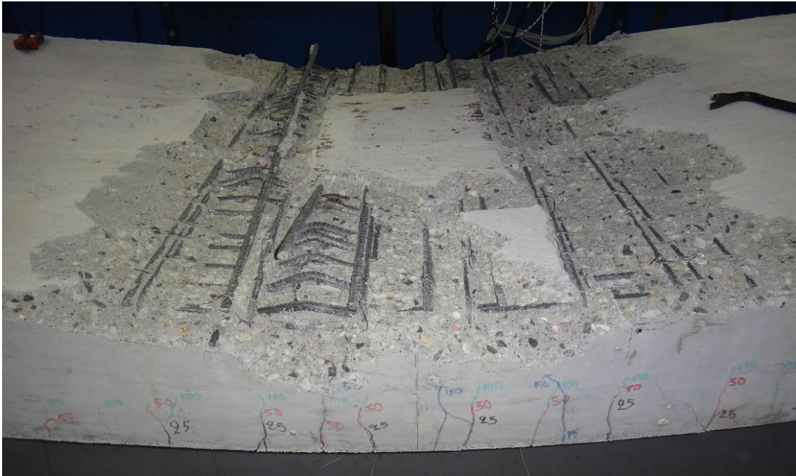
Fig. 5.115- S6b- The beam after the removal of loose concrete (fig. 5.117 and 5.118, points F and F')
