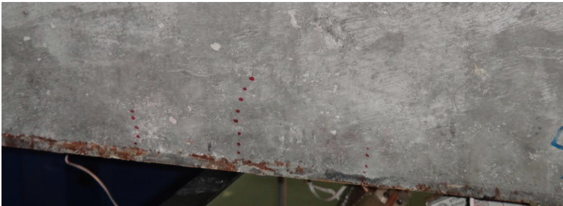
Fig. 5.50- S1- Hair-line cracks at deflection of 25 mm (fig. 5.57 and 5.58, points A and A')
