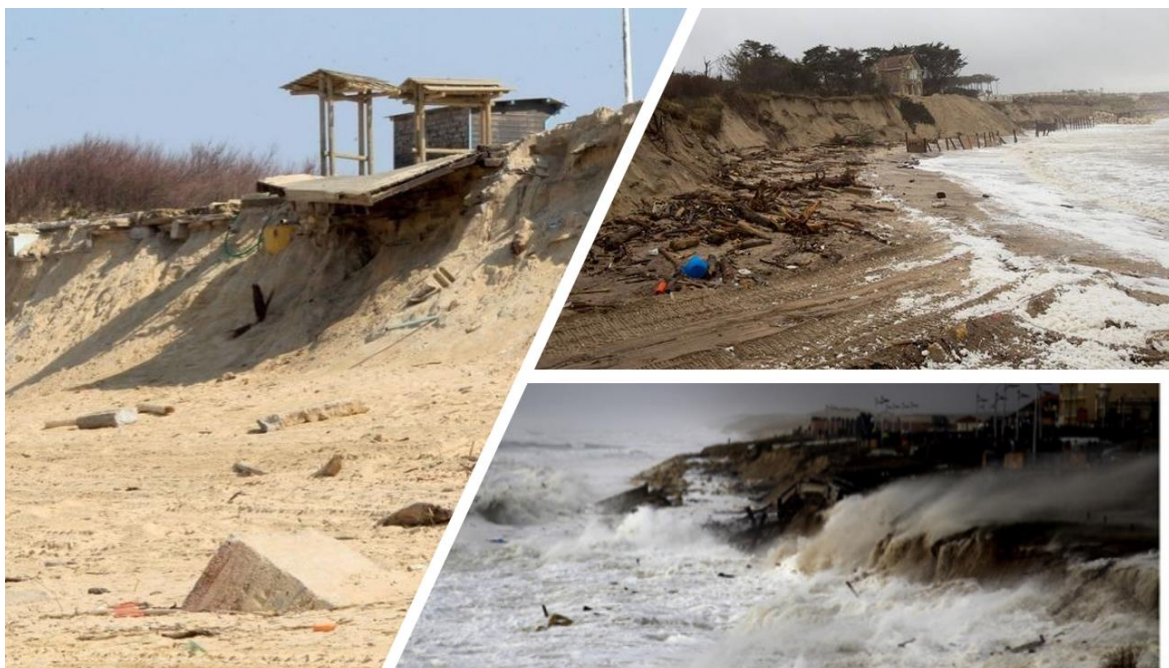
Figure 1-2 Images of the severe damaged sea defences and coastal erosion during the extreme storm events of the winter 2013/2014 in SW France.
