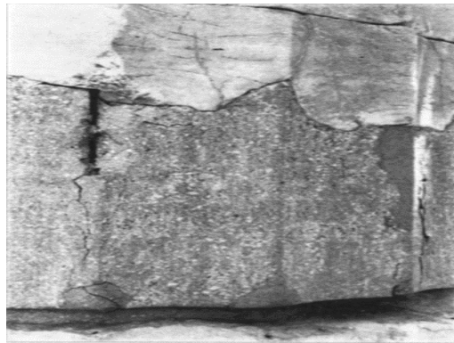
Figure 53: Marble breakage from a concrete reinforcement bar on BK 8, where BK stands for the north side column. (Study for the structural restoration of the northern side of the Parthenon, K. Zambas, YSMA 2002)
