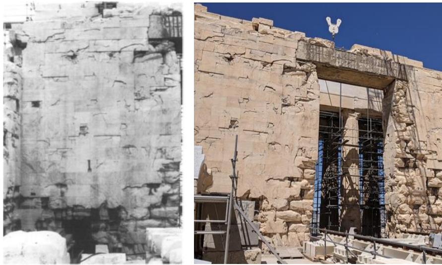
Figure 40: (left) The inner face of the West Door with extensive thermal fracturing observed on the plinths (Study for the restoration of the Parthenon, K. Zambas, vol.3b, YSMA 1994), (right) The preserved West Door.
