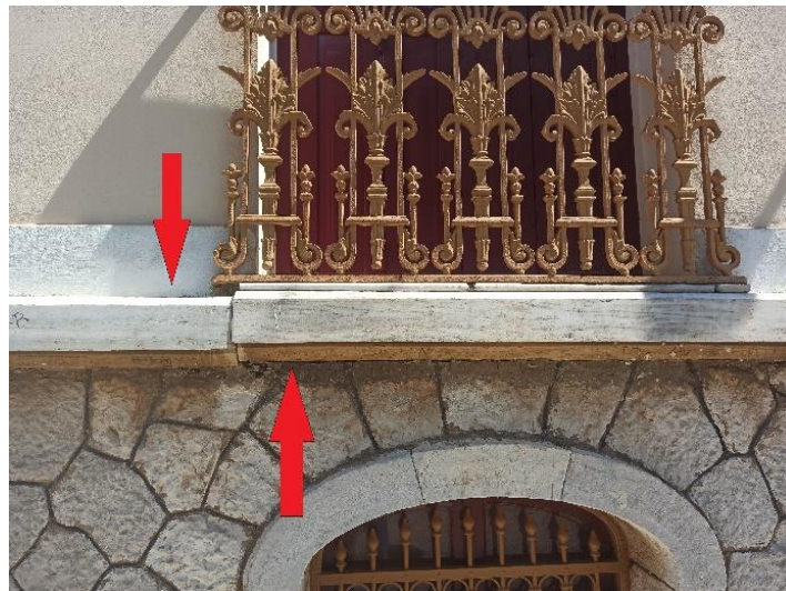
Figure 5. Damages recorded in buildings due to differential deformations. South side balcony damage in Building D
