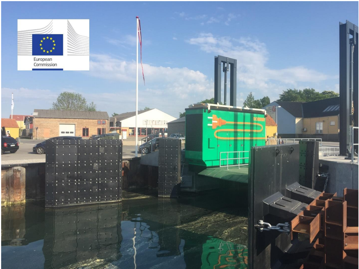
Figure 4. Port charging infrastructure for the E-ferry Ellen. (Source: http://e-ferryproject.eu/ . Accessed Jul. 15, 2023)
