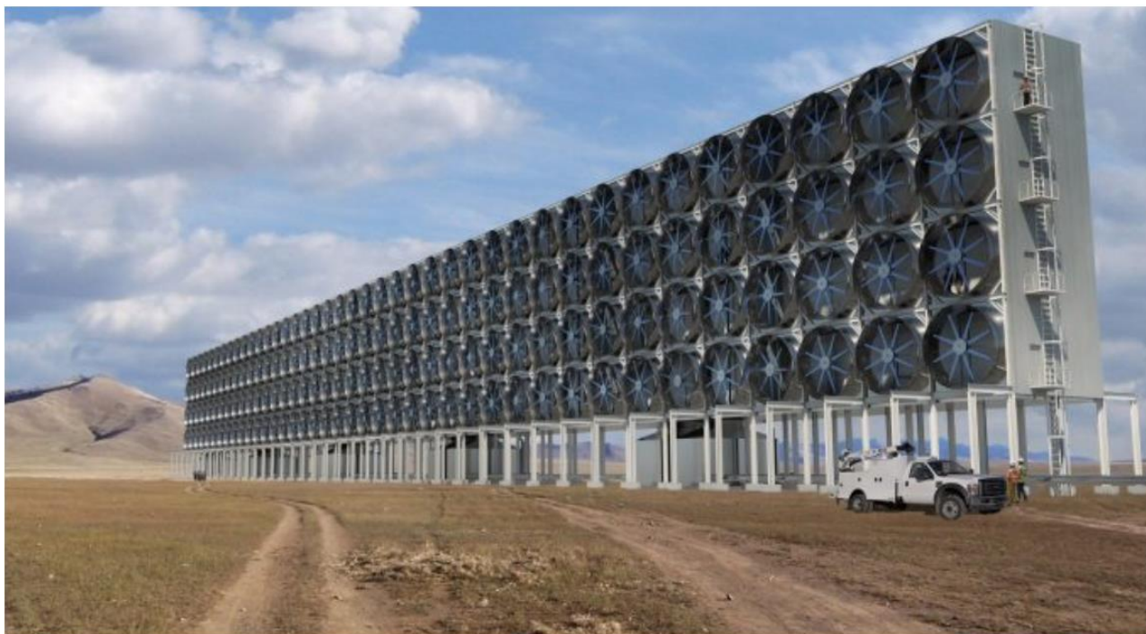
Carbon Engineering's large-scale CO 2 direct air capture plant at Squamish, British Columbia, CA ( Carbon Engineering Ltd. )
