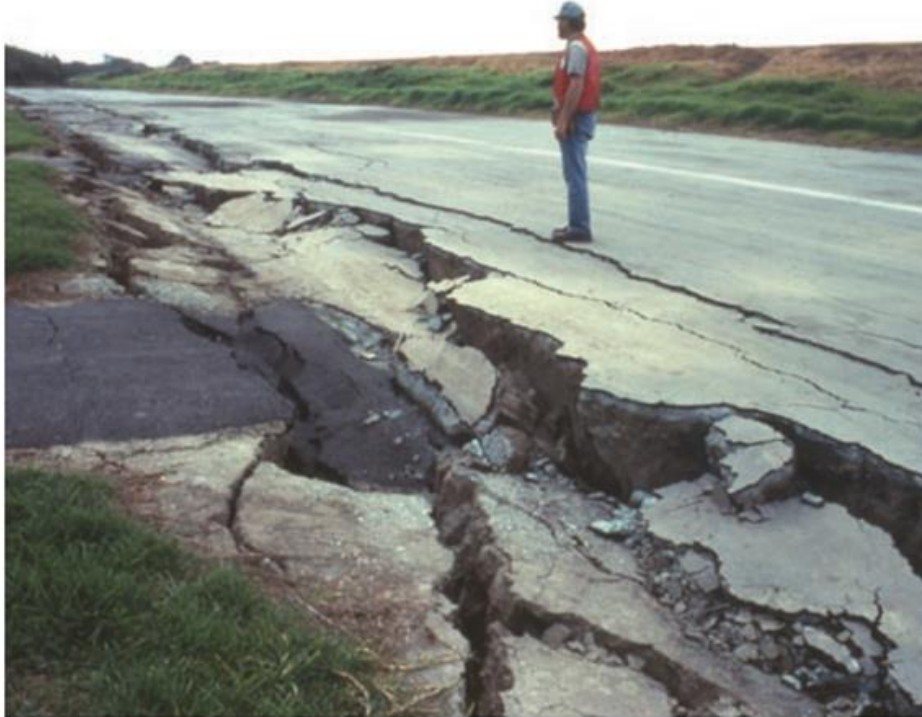
Photograph of lateral spread damage to a roadway as a result of the 1989 Loma Prieta, California, USA, earthquake. (Photograph by Steve Ellen, U.S. Geological Survey.)
