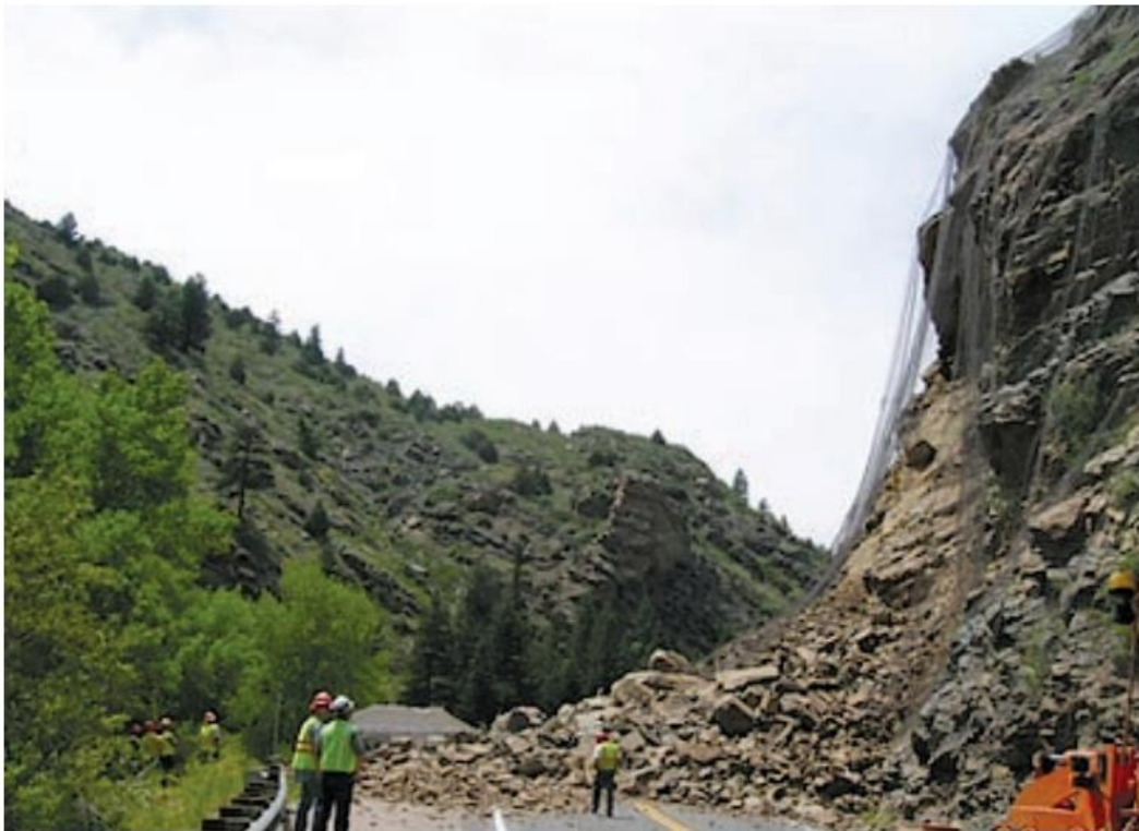
A rockfall/slide that occurred in Clear Creek Canyon, Colorado, USA, in 2005, closing the canyon to traffic for a number of weeks. The photograph also shows an example of a rock curtain, a barrier commonly applied over hazardous rock faces (right center of photograph). (Photograph by Colorado Geological Survey.)
