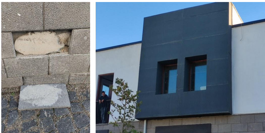
Figure 8.19. Poor materials/workmanship: stone cladding is already collapsing, and black walls are fading (taken by the author, 2022).
