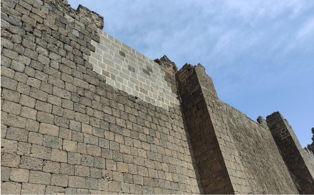
Figure 8.31. Poor restoration to historical wall; foreign architectural elements cause inaccurate match and disrupt overall coherence (taken by the author, 2022).
