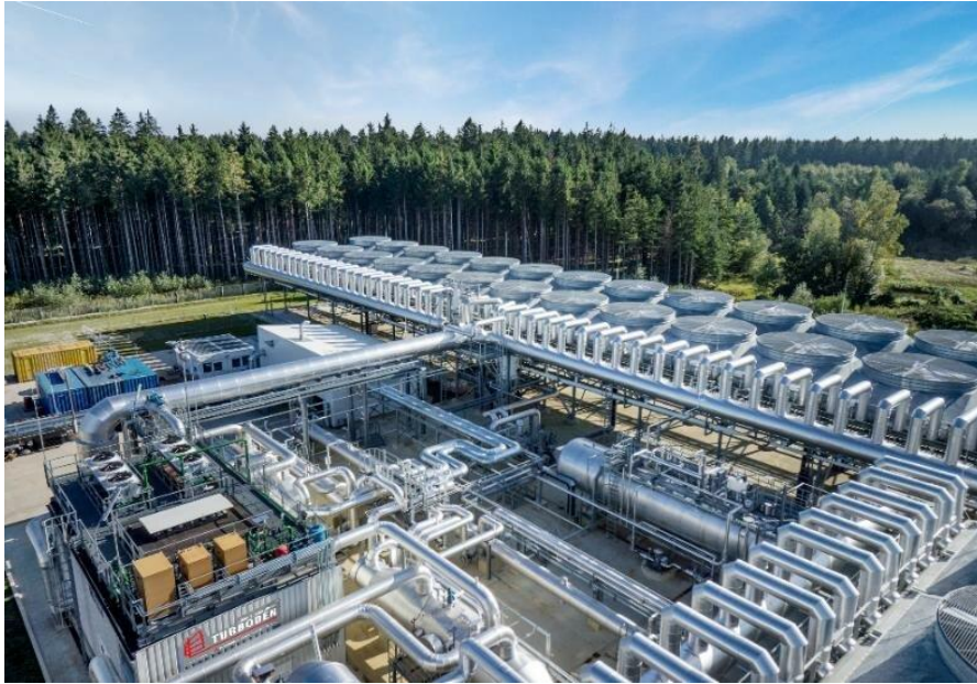
Figure 1.15 :6 MWe ORC installation with the air-cooled condenser in Germany [39]
