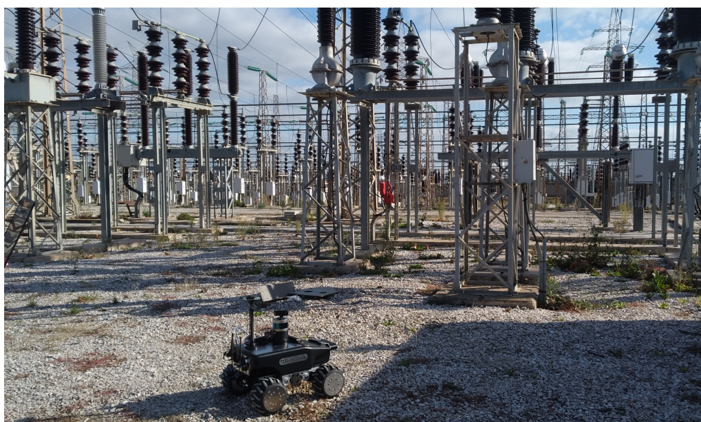
Figure 4.2. Our mobile robot in the high voltage facility
