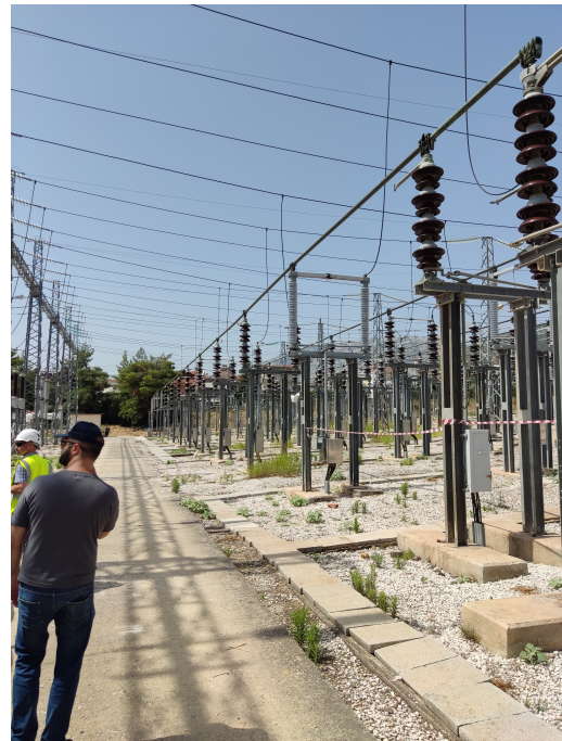
Figure 1.2. High voltage facility, some elements that may need inspection shown.
