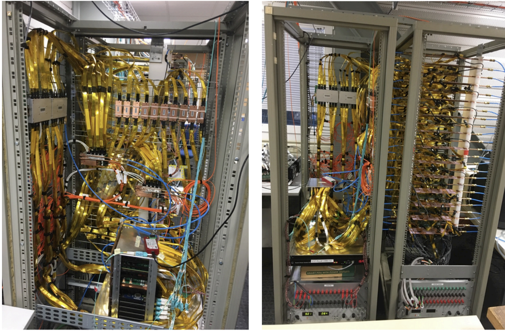
Figure 4.59: The NSW electronics setup at the Vertical Slice laboratory.
