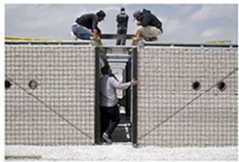
RE-BUILD (2015) | Pitosio Building Peace Organization, Pouya Khazaeli, Cameron Sinclair 01_Α | 02_Ε | 03_Α | 04_Ε | 05_Β | 06_Ε | 07_Β | 08_Ζ | 09_Α | 10_Ε
