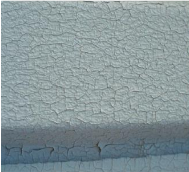
Figure 69: Cracking (2) (PST, Photo Gallery, 2015)
