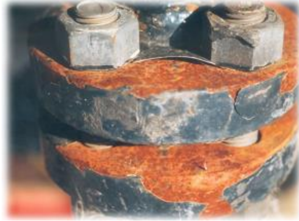
Figure 60: Adhesion Failure (PST, Photo Gallery, 2015)
