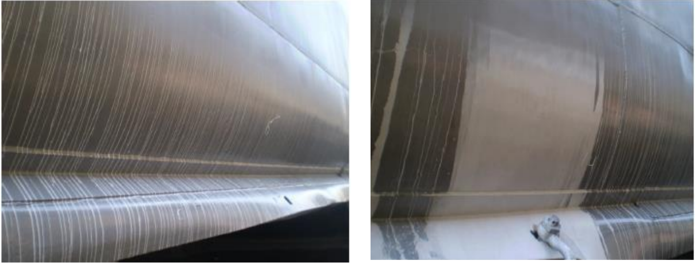
Figure 80: Water leaking on the wet paint film which resulted to blushing (PST, Photo Gallery, 2015)
