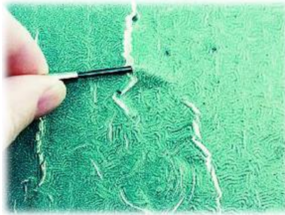
Figure 68: Cracking (PST, Photo Gallery, 2015)
