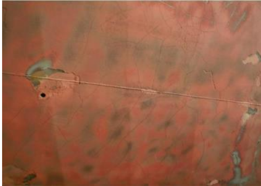
Figure 70: Cracking (3) (PST, Photo Gallery, 2015)
