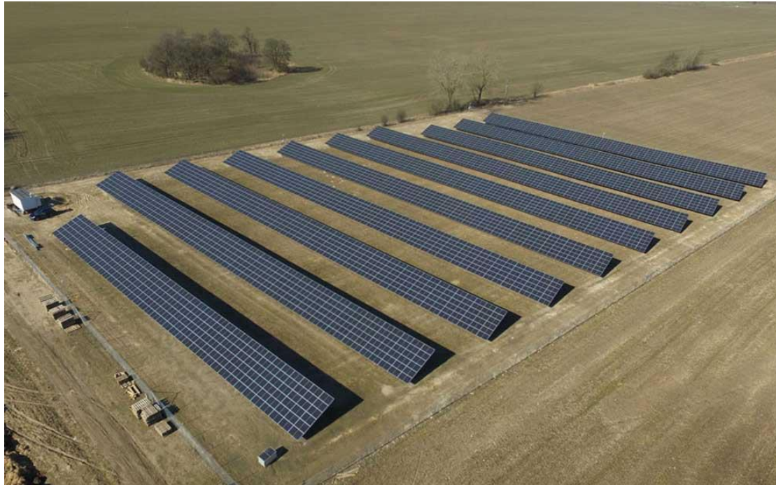
Figure 2: Example of 1MW PV Park
