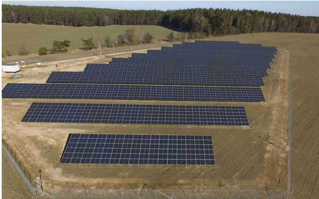
Figure 1: Example of 1MW PV Park
