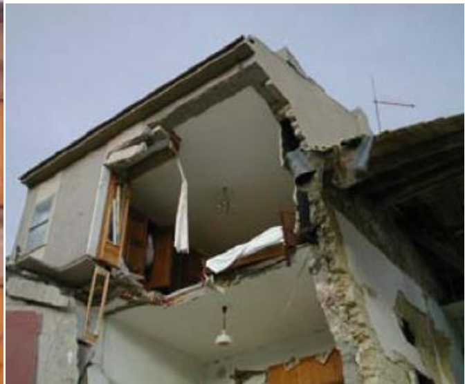
Fig. 18 Typical failure due to inadequate stiffness of the wall (d) (from E. Vintzilaïou – “Lecture notes on Advanced Mechanics of Masonry”)
