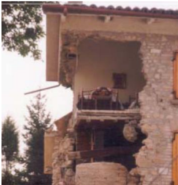
Fig. 17 Typical failure due to inadequate stiffness of the wall (c) (from E. Vintzilaïou – “Lecture notes on Advanced Mechanics of Masonry”)
