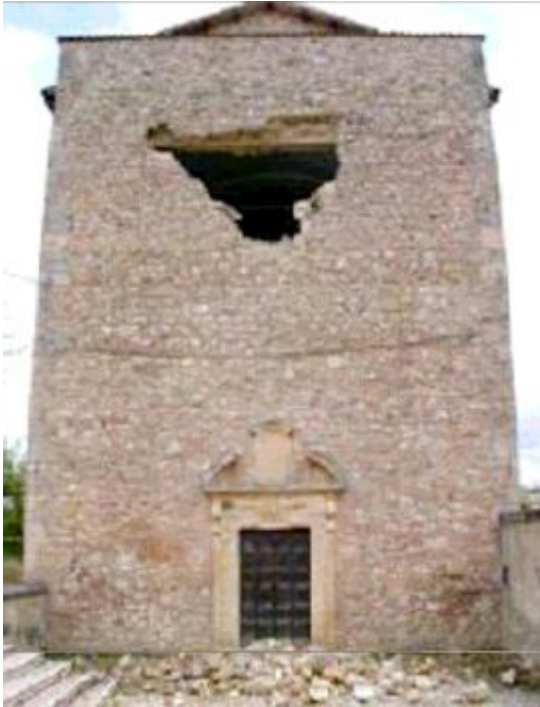
Fig. 15 Typical failure due to inadequate stiffness of the wall (a) (from E. Vintzilaïou – “Lecture notes on Advanced Mechanics of Masonry”)
