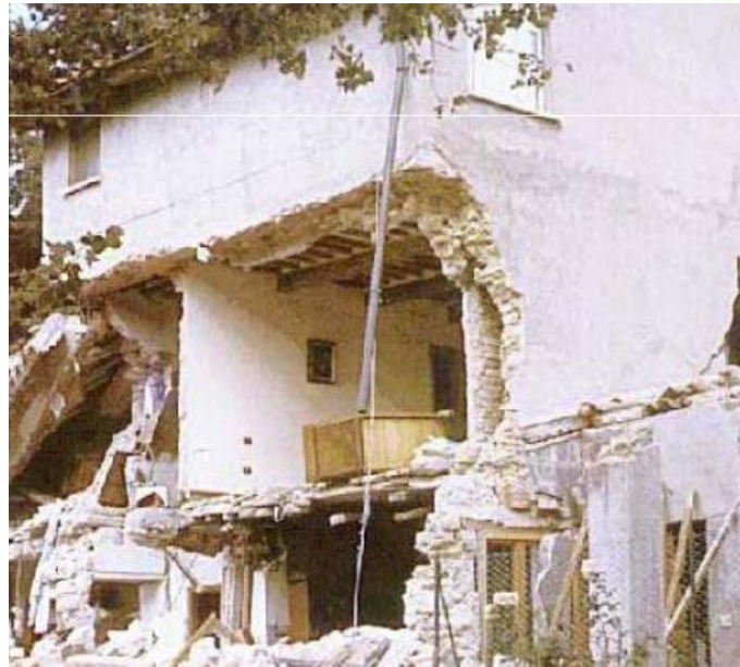
Fig. 16 Typical failure due to inadequate stiffness of the wall (b) (from E. Vintzilaïou – “Lecture notes on Advanced Mechanics of Masonry”)
