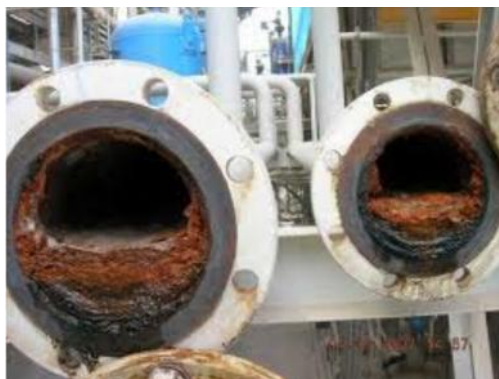
Figure 22 : Pipe Corrosion and Fouling
