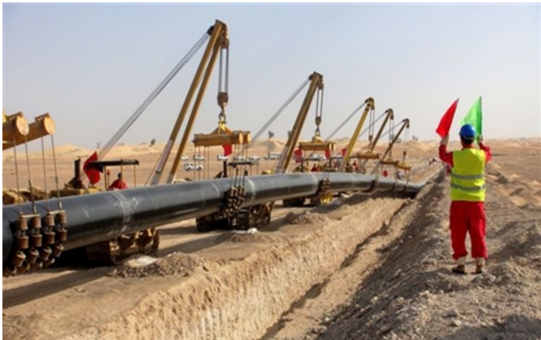
Figure 1.3.5. Pipe-laying process of the 370km Fujairah oil pipeline in the United Arab Emirates ( www.pipelinesinternational.com ).
