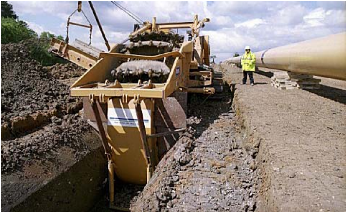
Figure 1.3.3. Excavating pipe trench using trenching machine (Lincolnshire gas pipeline works, United Kingdom).
