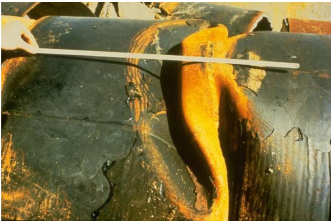
Figure 1.5.10. Wrinkled pipeline failed in compression (Takada et al.2001).
