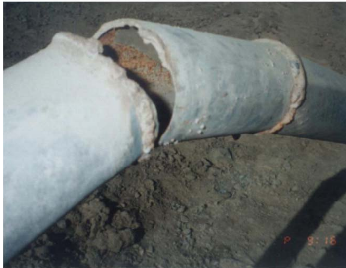
Figure 1.5.7. Fault-induced damage of embedded pipeline during the Manjil earthquake 1990, Iran (Sim et al.2012).
