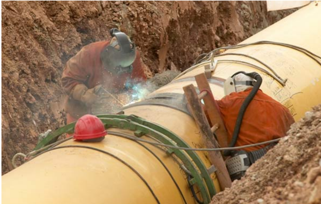
Figure 1.3.6. Welding process. South Wales gas pipeline. UK's largest high-pressure gas pipeline (317 km) ( www.nationalgrid.com ).
