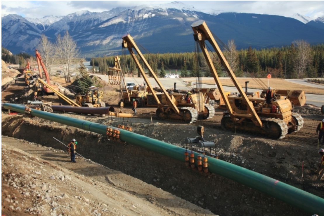
Figure 1.3.4. Laying down the gas pipeline that runs from Edmonton to Vancouver, Canada (Canadian Energy pipeline Association).
