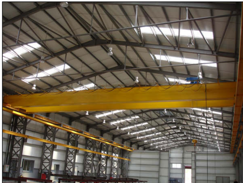
PICTURE 1.1-EXAMPLE OF OVERHEAD CRANE
