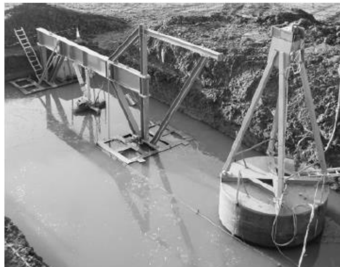
Figure 6-2: The 3 meters diameter suction caisson that was subjected to dynamic loading in the field.
