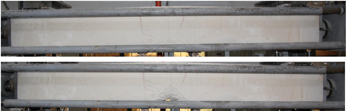
Figure 5.9: Crack pattern of the fifth beam.
