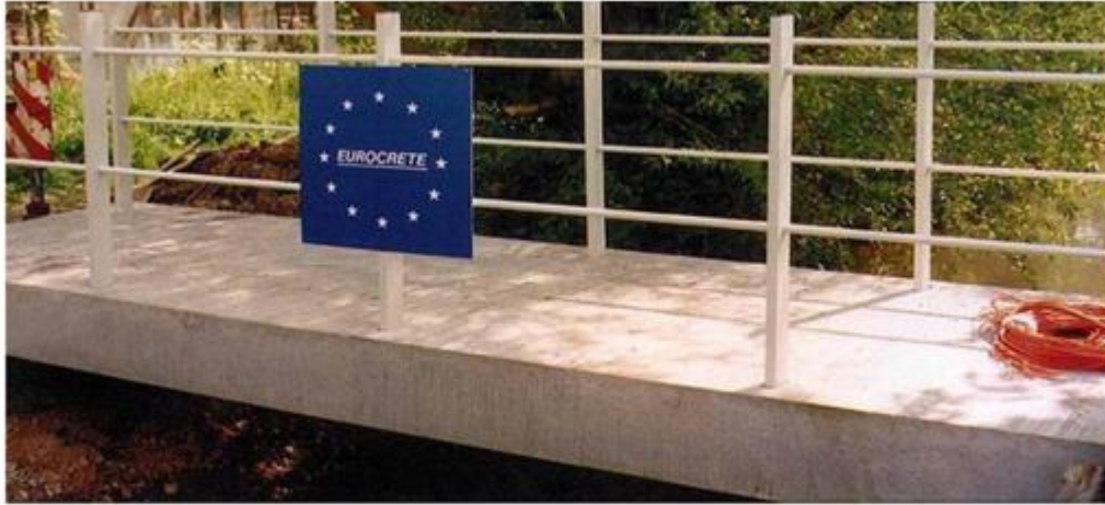
The first concrete footbridge in Europe with only FRP reinforcement (EUROCRETE project,
