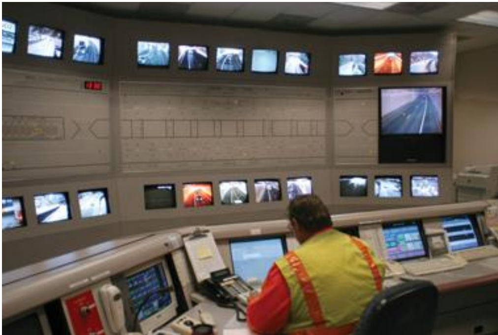
Figure 7: A road tunnel operator (PIARC 2008b)
