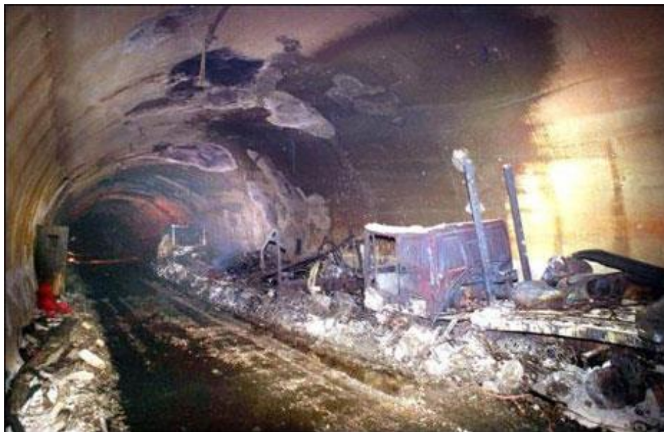
Figure 2: Consequences of the Mont Blanc tunnel fire (Lacroix 2001)
