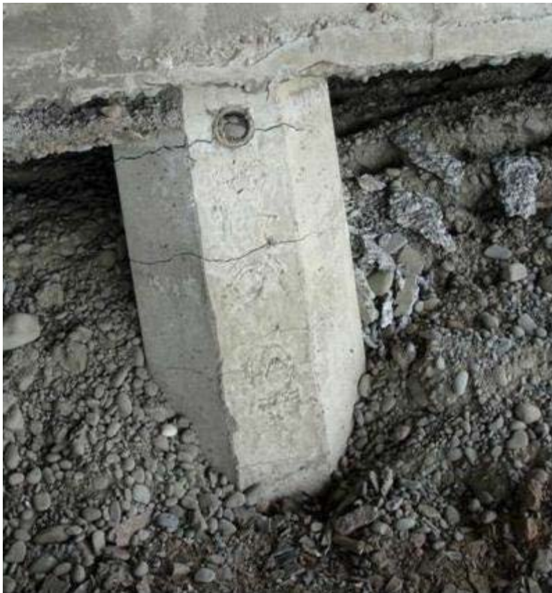
Figure 1.14: Western abutment of South Bridge Road Bridge after Christchurch earthquake: (a) Concrete spalling exposing the pile reinforcement, (b) Flexural cracks developed at the top of the piles indicating plastic hinging (Tasiopoulou et al, 2011)
