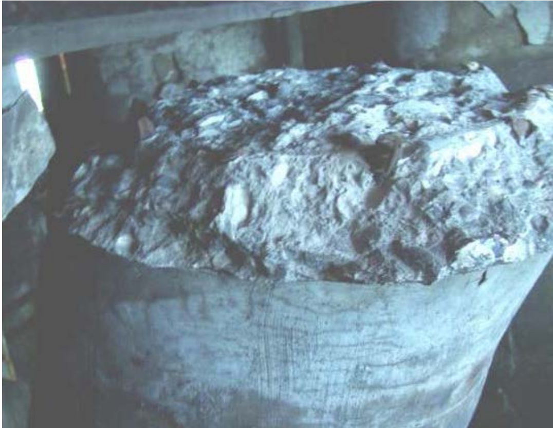
Figure 1.13: Broken pile cap in a wharf extension during the Chile 2010 earthquake (Villalobos et al, 2011)
