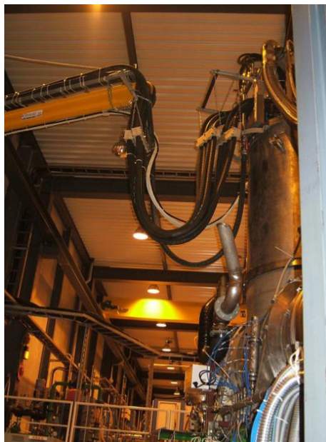
Picture 3.4: The cables connected to the magnet, surrounded by a cooling system.
